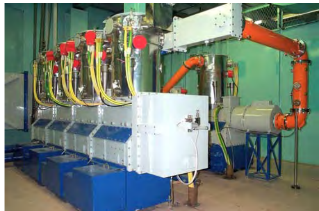
Fig.5: RF generator, general view
