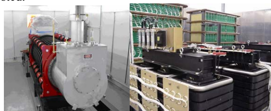
Figure 1: a. (left) the CPI klystron. b. (right) the 95kV 20A DRC power supply.
