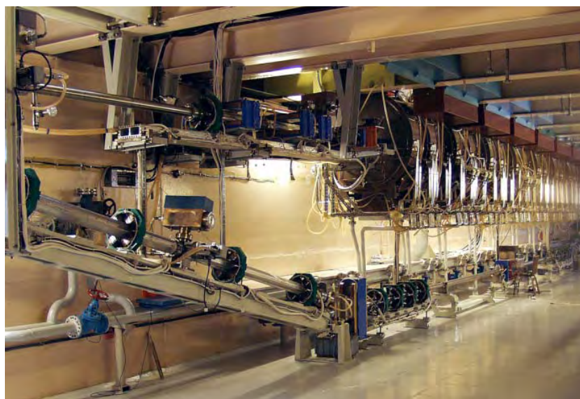
Fig. 3 General view of the Novosibirsk terahertz FEL (NovoFEL).
