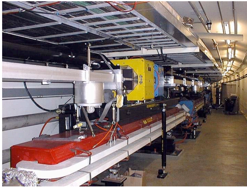
Figure 1: PEP-II tunnel with LER above the HER.
