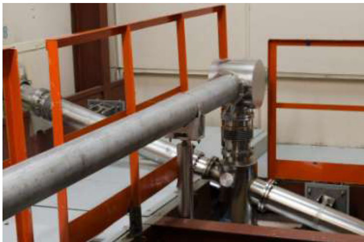
Fig. 4. Optical beamline for FELs. Radiation of all FELs is delivered to the same user stations. Switching between FELs is done using retractable mirrors.
