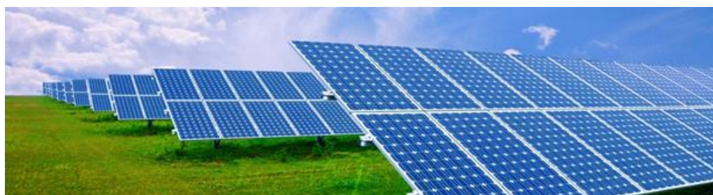
Fig. 1. Solar power plant.
