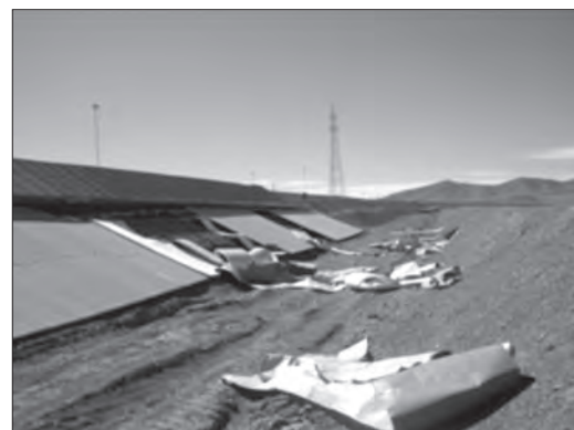
Fig. 2. Scene after sun-shading board destroyed in winter in Qinghai-Tibet railway.
