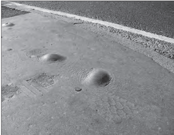
Fig. 1. Asphalt blisters on pavements of London.
