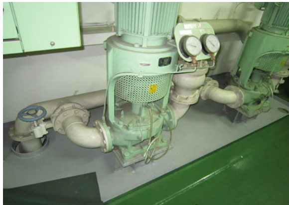
Fig. 22.3 Pipes connecting two vertical centrifugal pumps in a ship engine room
